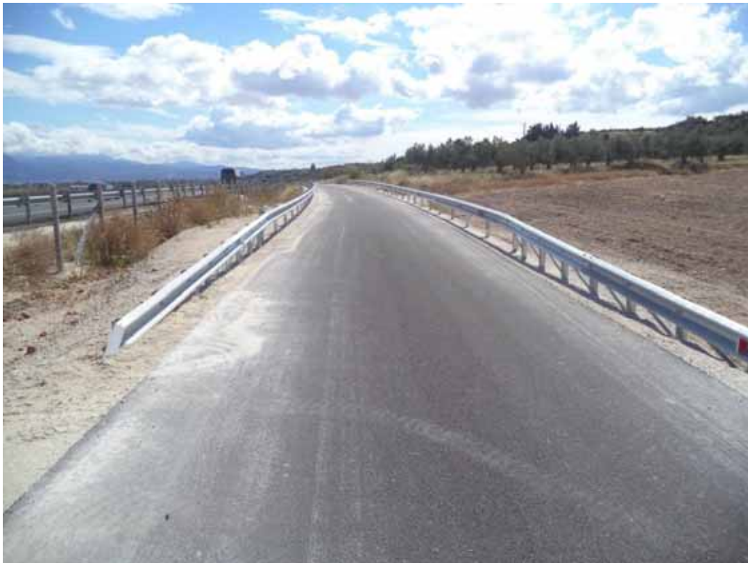
Safety barriers at SR 004L
