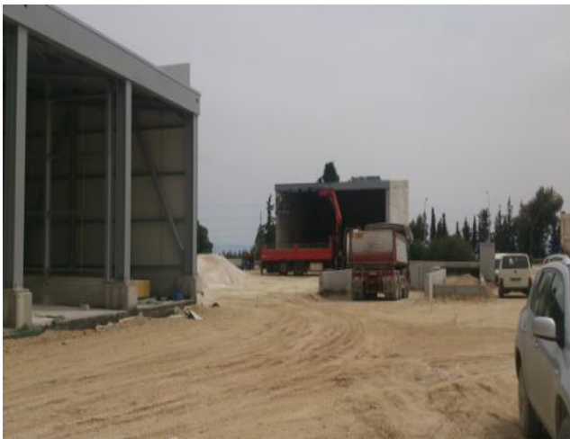
Installation of metal frame at Salt Shed (Y169) of Kiato Technical Base
