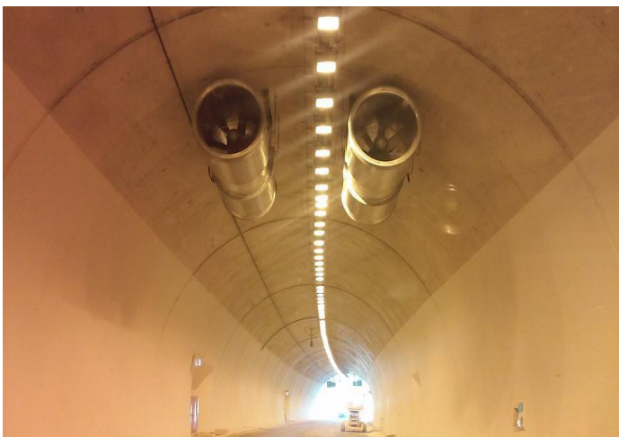
Tunnel Akrata 13A – Ventilation system
