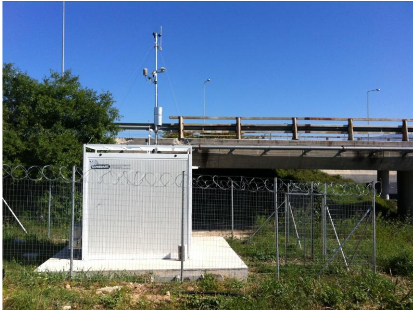
The environmental station at Tripoli Semi-I/C
