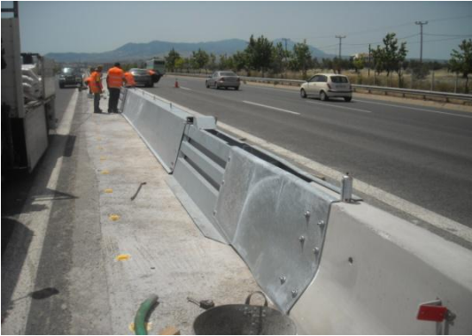
Safety works – Placement of door at the Emergency Median Opening at k.p. 43+100
