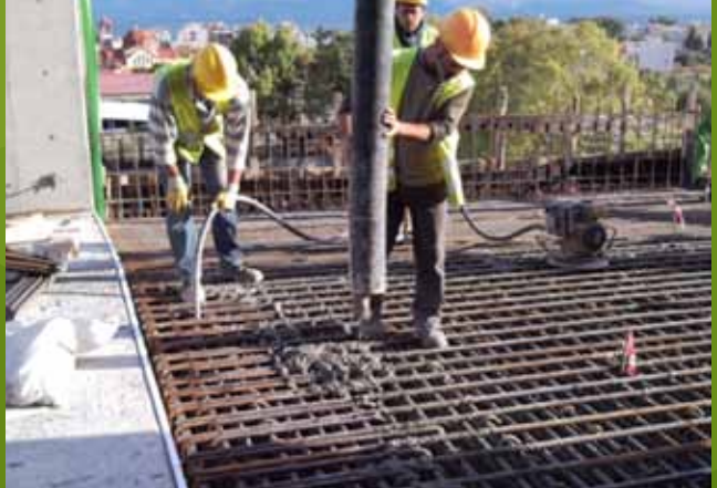
Xylokastro Lane Cover C003: Pouring of 2nd phase of top slab, segment 3
