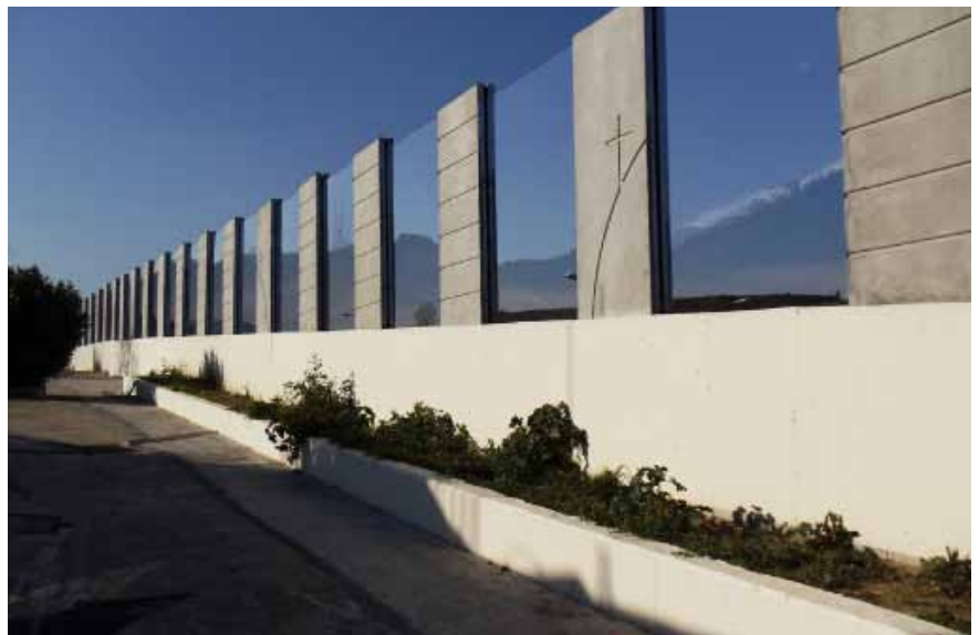
Installation of sound barriers, in the Project's existing sections (Zoodochos Pigi Abbey, Patra By-Pass)
