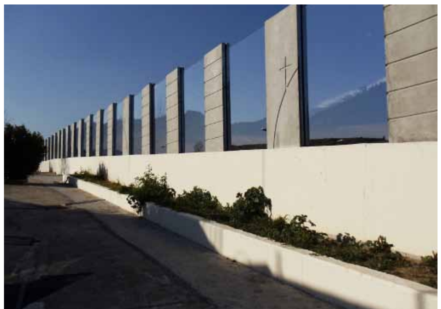
Installation of sound barriers, in the Project's existing sections (Zoodochos Pigi Abbey, Patra By-Pass)
