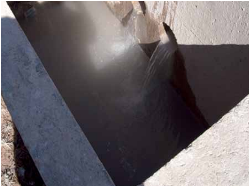
Sedimentation tank in Panagopoula tunnel
