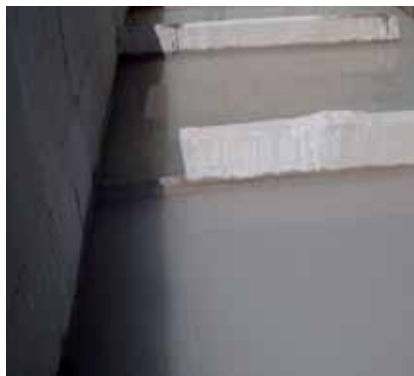
Sedimentation tank in Panagopoula tunnel
